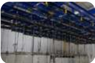
Multi-track transfer carriage
